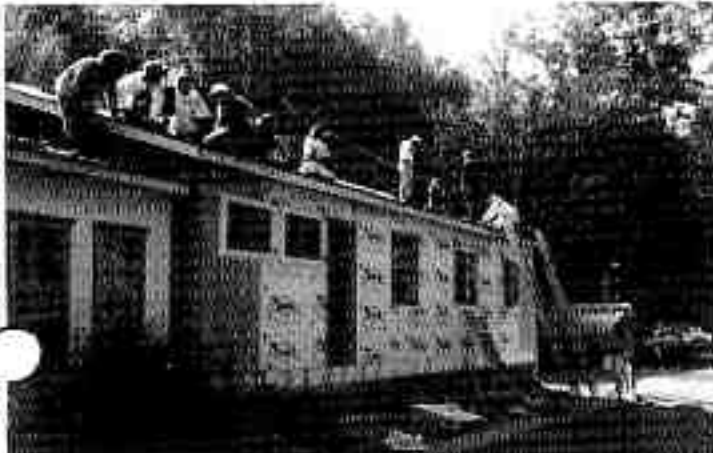
Volunteers nail shingles and snap lines on the third day of the blitz build.
